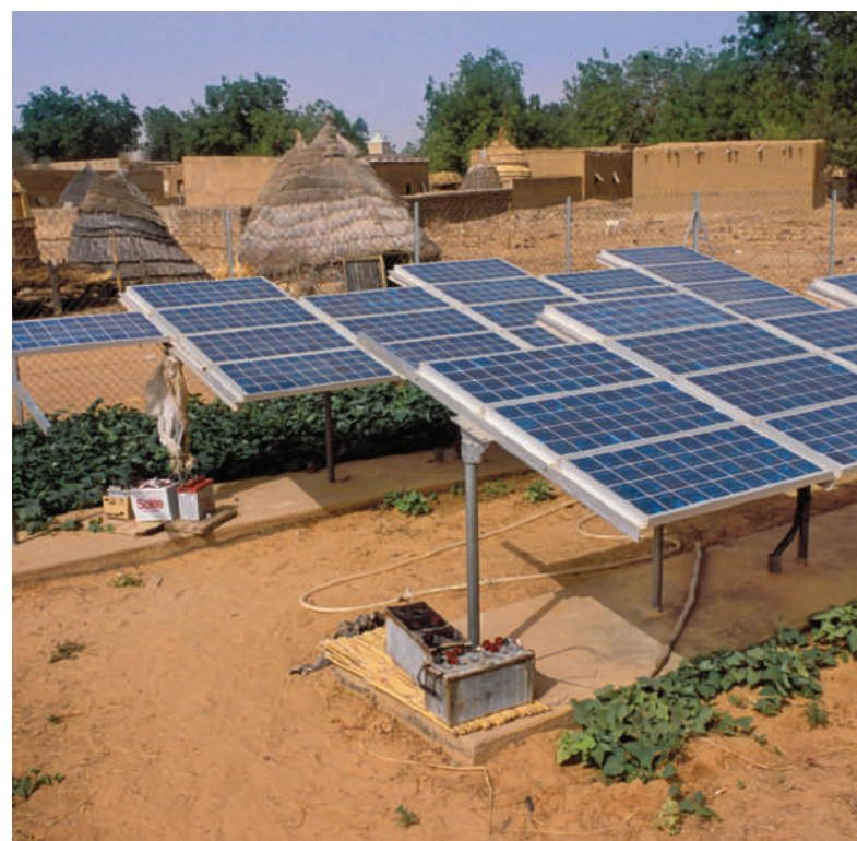
Figure 16-18 Solutions: solar cells used to provide electricity for a remote village in Niger, Africa. Question: Do you think your government should provide aid so poor countries can obtain such solar cells? Explain.
